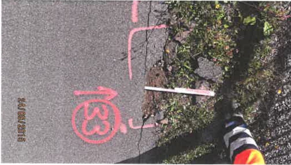
Punkt 33 = 16cm (Risse)
