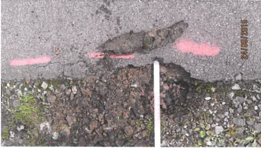
Punkt 30 = 5cm (Risse)
