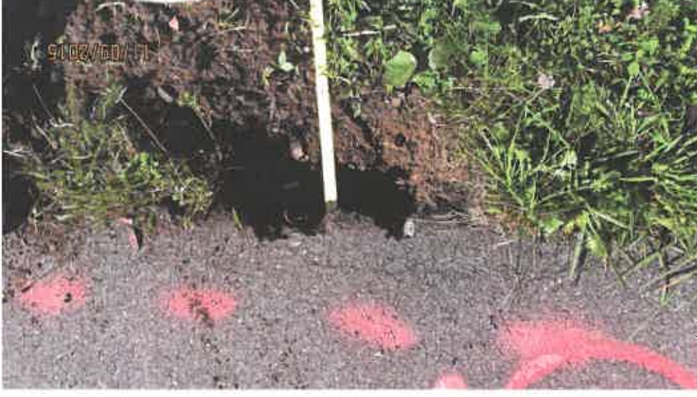
Punkt 12 = 6cm (Risse)
