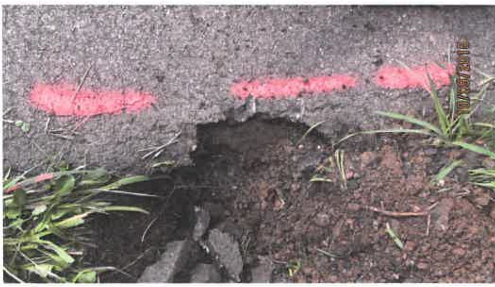
Punkt 1 = 3cm (Risse)
