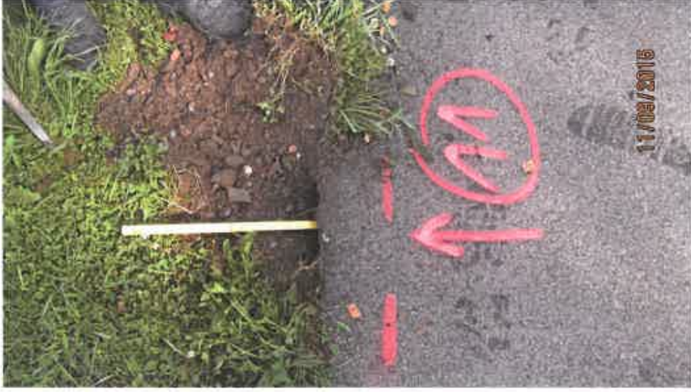
Punkt 11 = 5cm (Risse)
